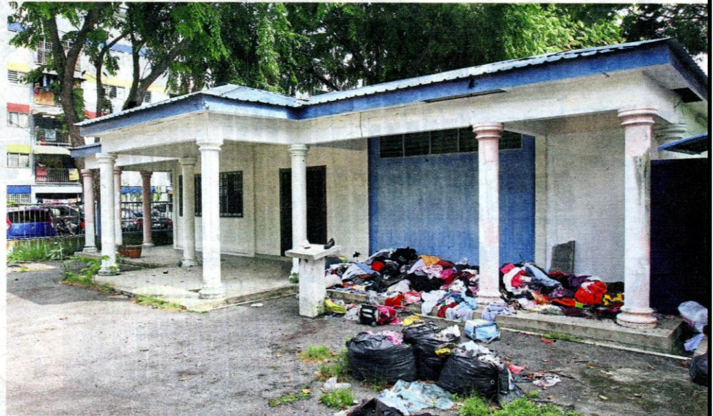
A community hall in Bandar Tun Razak near Jalan Ikan Emas is abandoned and in a deplorable state.
