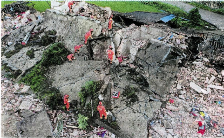
Rescue workers searching the rubble of a collapsed building in Yibin, Sichuan province, yesterday. REUTERS PIC
